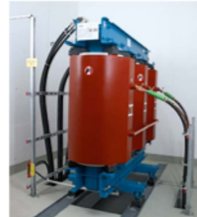
Rectifier transformer by Siemens.
