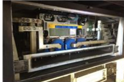
Inverter Installed on a Train Courtesy of MBTA.
